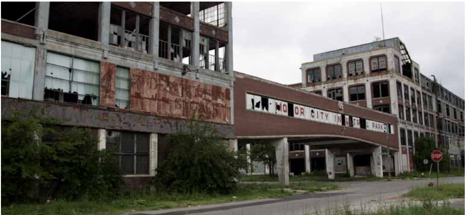
SHUTTERED: The abandoned and decaying Packard Motor Car Manufacturing plant, built in 1907 and designed by Albert Kahn, is seen near downtown Detroit, Michigan June 21, 2009. REUTERS/REBECCA COOK
