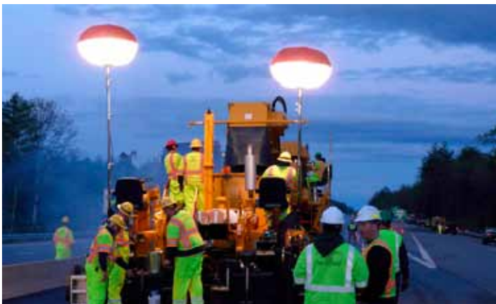
HIT THE ROAD: New Hampshire started the Route 101 project to create jobs for construction and stimulate the state's economy. Exeter, New Hampshire June 3, 2009. REUTERS/HO NEW
